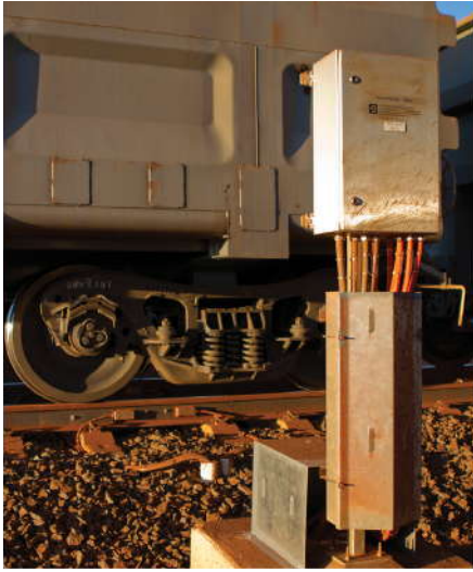
Meridian track scale for tare weighing at Christmas Creek.
